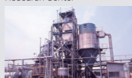
Diallyl phthalate (DAP) resin production facility
