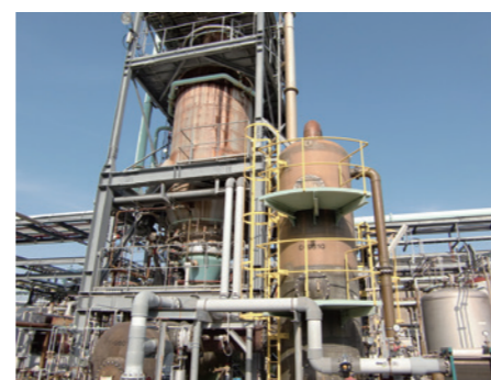
Facility for recovery of valuable materials through thermal decomposition of wastewater (Matsuyama Plant)
