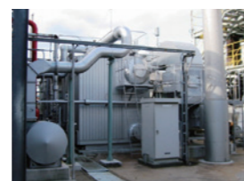
Hydrogen boiler (Matsuyama Plant)
