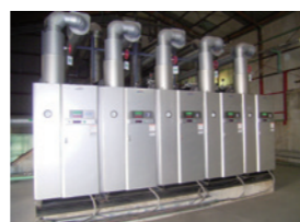
City gas boilers (Amagasaki Plant)
